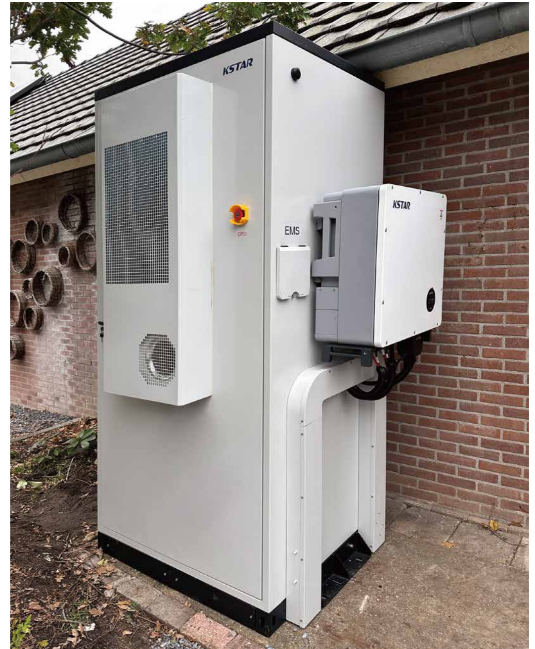
03 C&I ESS Project in the Netherlands
