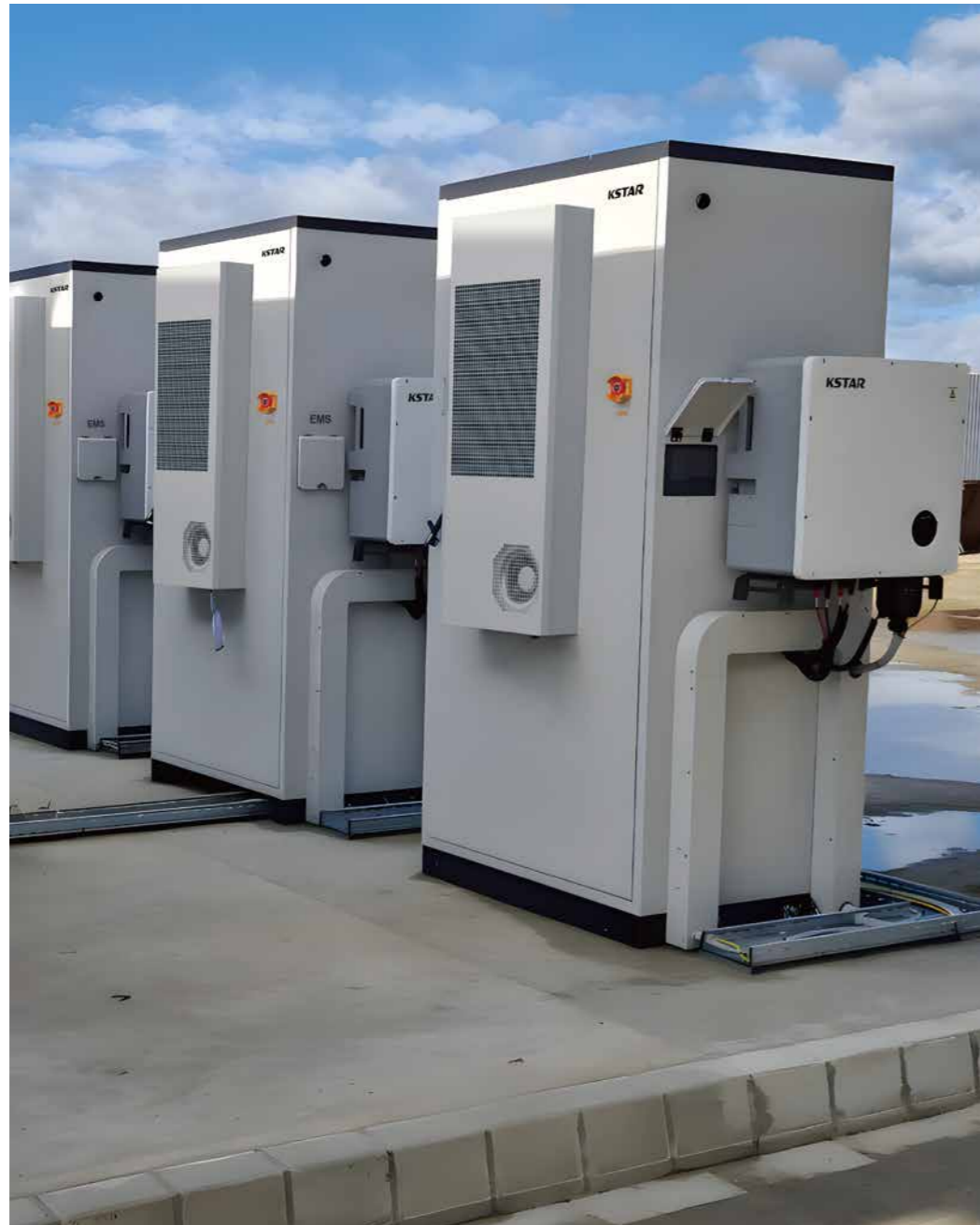
02 C&I ESS Project in Hungary
